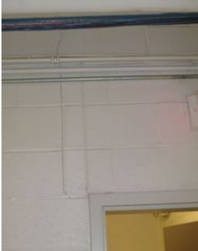
Cracking is present over this door frame in the basement.
