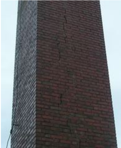
Cracks and mortar wash-out are visible on this chimney
