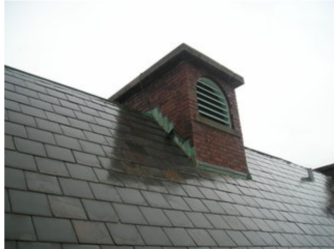
Flashing is damaged at this dormer
