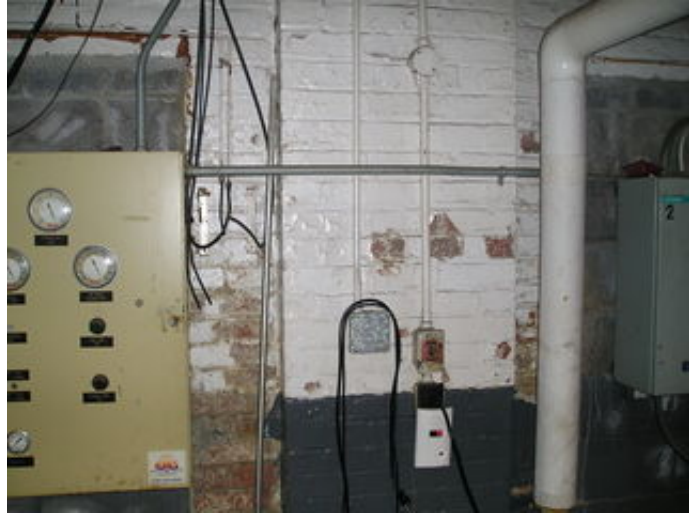
Evidence of water breach is seen at this basement wall.
