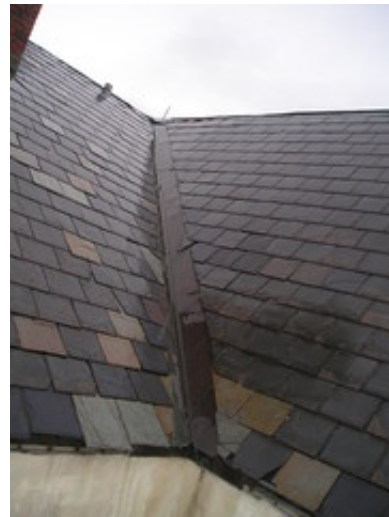
Damaged and replaced slate near valley
