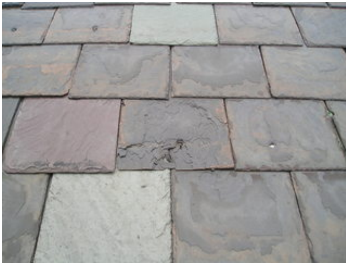
Damaged and replaced slate tile
